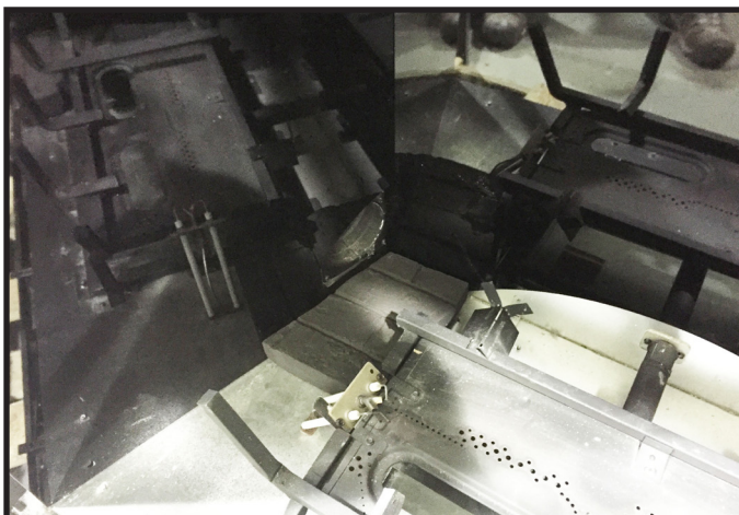
Figure 14 Left Rear Base Refractory
